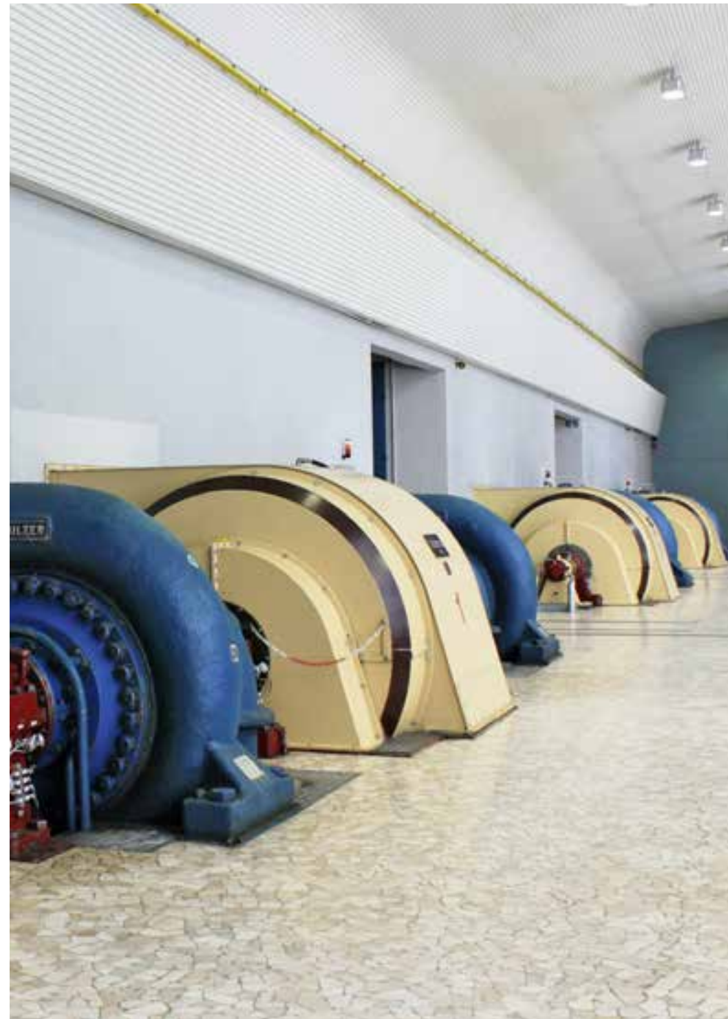
Arolla pumping station machines room
