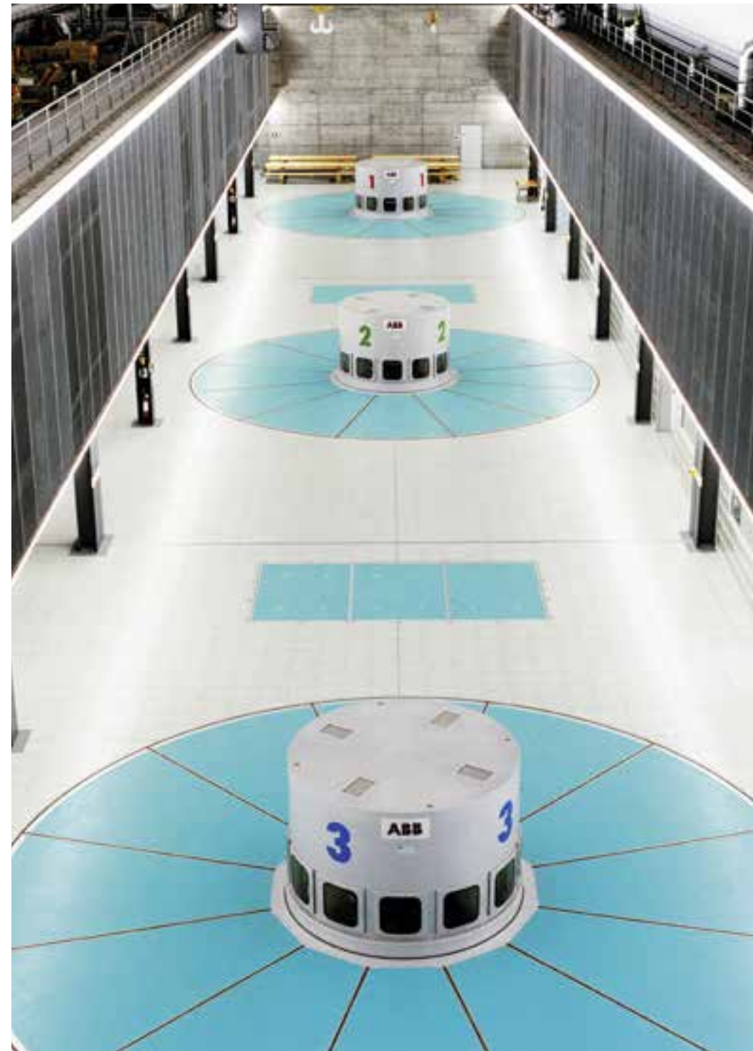
Machines room, Bieudron power plant
