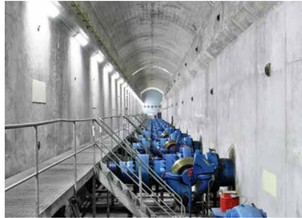
Valves chamber, Nendaz power plant
